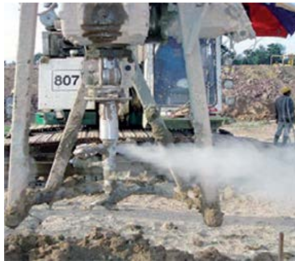
Figure 12: Injection of dry binder into the soil from the mixing tool (Keller)
