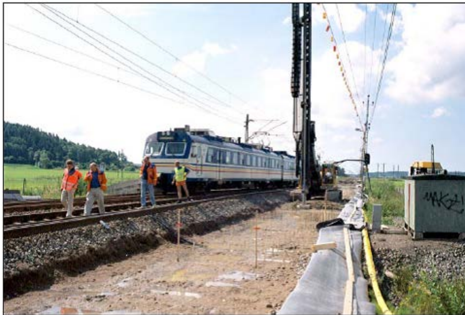
Figure 22: Vibration mitigation using Dry deep mixing method; column installation in progress while commuter train passing (Holm et al, 2002)
