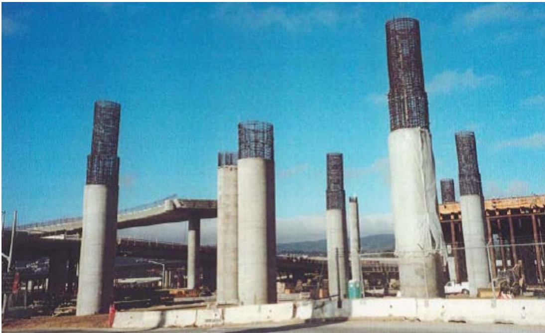
Figure 14: Railroad Bridge supported by deep mixing column at San Francisco International Airport (Porbaha et al, 2005)
