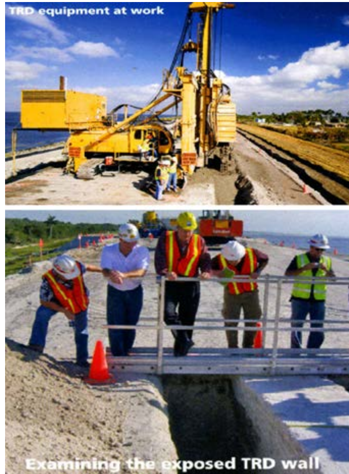
Figure 17: Top: TRD equipment at work, Bottom: Inspection of the exposed TRD wall at Herbert Hoover Dike surrounding Lake Okeechobee in southeastern Florida (Hayward Baker Inc.)
