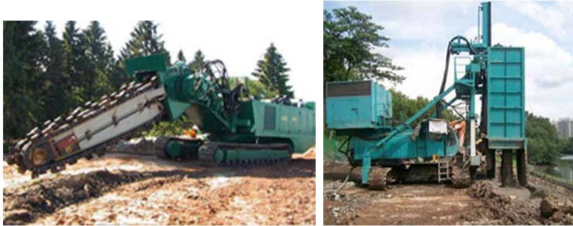
Figure 5: The FMI and TRD–Trenching machine for construction of deep walls (Massarsch and Topolnicki, 2005; Hayward Baker Inc.)
