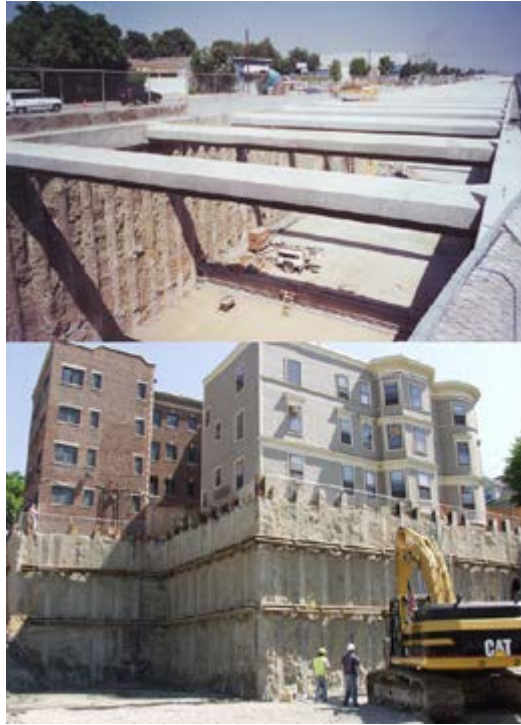
Figure 19: Top: Trench excavation railroad for an Alameda corridor project. Bottom: Structural cutoff wall during construction of new facility at Harvard University, Cambridge (Porbaha et al, 2005)
