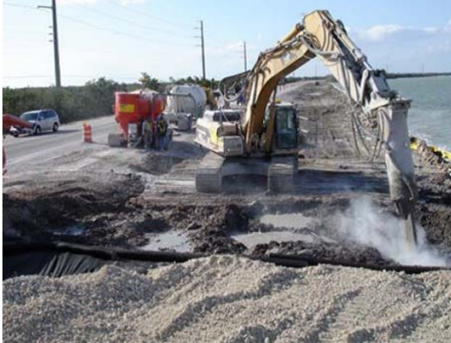
Figure 27: Dry mass soil mixing to strengthen soft soils beneath a planned roadway expansion at U.S. Highway 1, Key Largo, Florida (Hayward Baker Inc). Geo-fabric separate placed on top of stabilized mass before the selected base coarse layer is placed.
