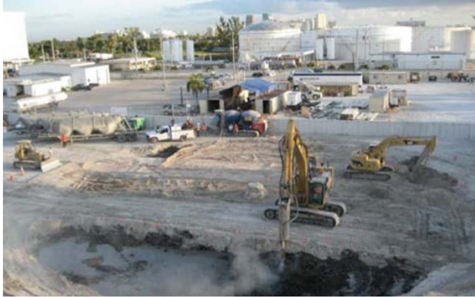
Figure 28: Mass stabilization with dry soil mixing of soft wet organics to control settlement for storage tanks at Port Everglades, Florida (Haward Baker Inc.)
