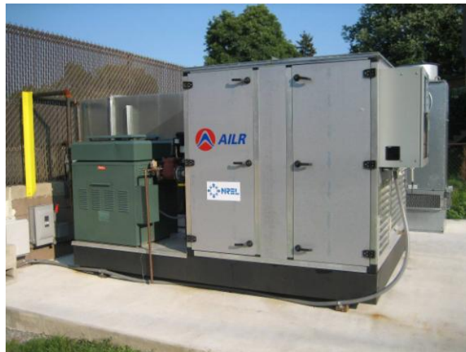
Figure 8. The second prototype of a low-flow LDAC processing ventilation air for a machine shop in Wrightsville, Pennsylvania.
