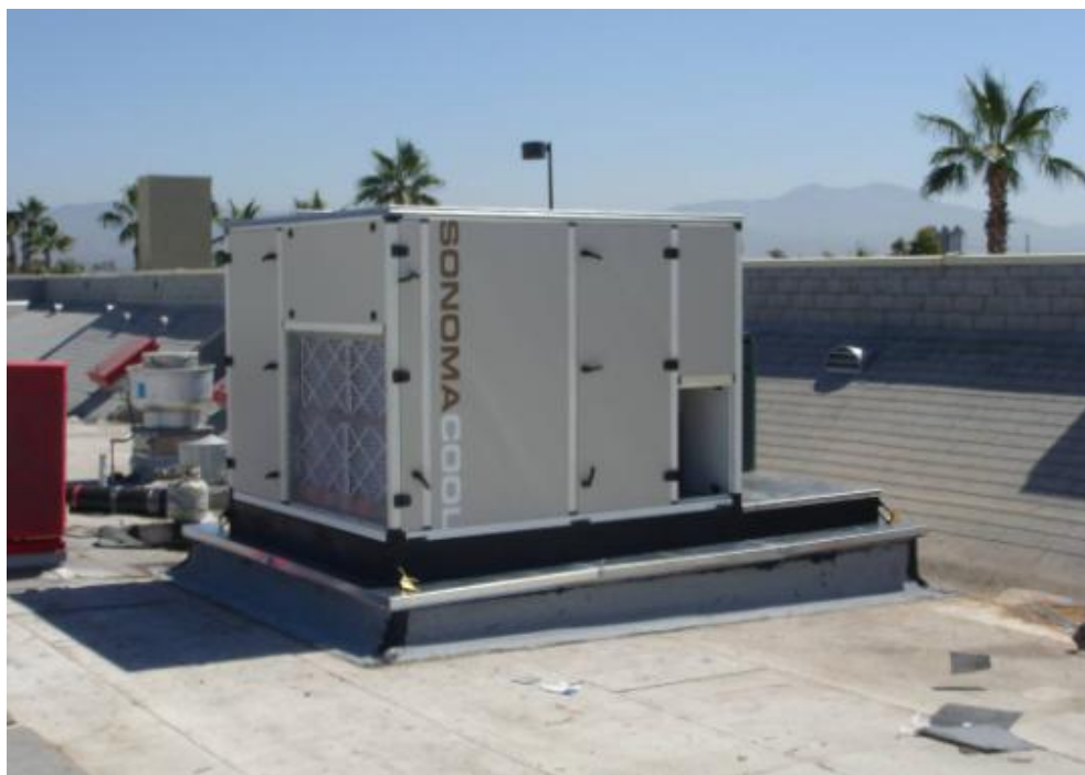
Figure 9. Commercial LDAC using low-flow technology installed on a Los Angeles supermarket.
