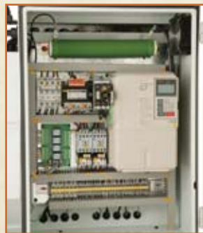
YASKAWA FREQUENCY DRIVE AND ALLEN-BRADLEY® CONTROLS
