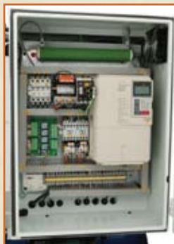
YASKAWA FREQUENCY DRIVE AND ALLEN-BRADLEY® CONTROLS
