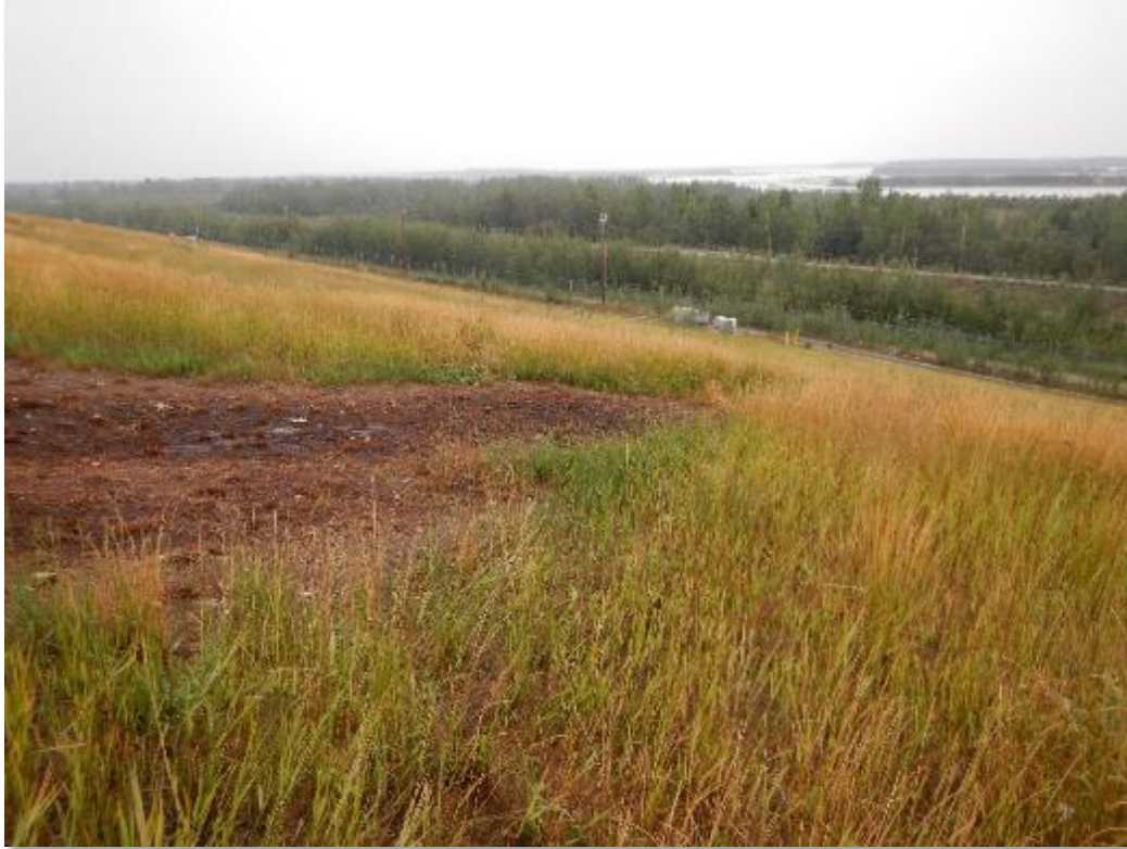
Orange staining and dead vegetation characteristic of a leachate seep.
