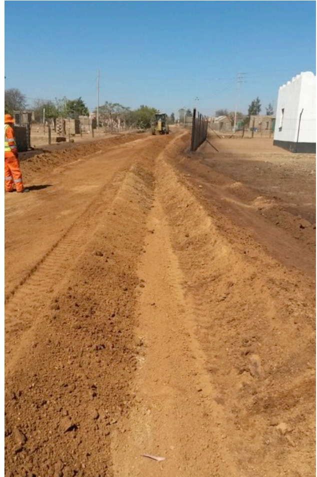
(4) The windrows are moved across the road while GreenBit is sprayed to ensure an even mix.
