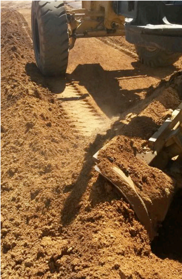
(3) A grader is used to mix the GreenBit product with the road material.
