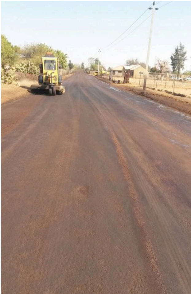
(7) The road is sealed using a mechanical sweeper to remove loose material and to ensure a good seal.
