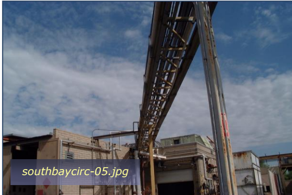
Photo #3: Overhead Piped Delivery to the IWTP Taken By: Greg V. Arthur Date: 08/11/09
