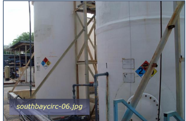
Photo #4: IWTP Incoming Equalization Tanks Taken By: Greg V. Arthur Date: 08/11/09
