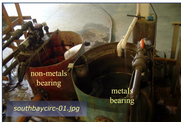
Photo #1: Main Bldg 6409 Transfer Holding Tanks Taken By: Greg V. Arthur Date: 08/11/09
