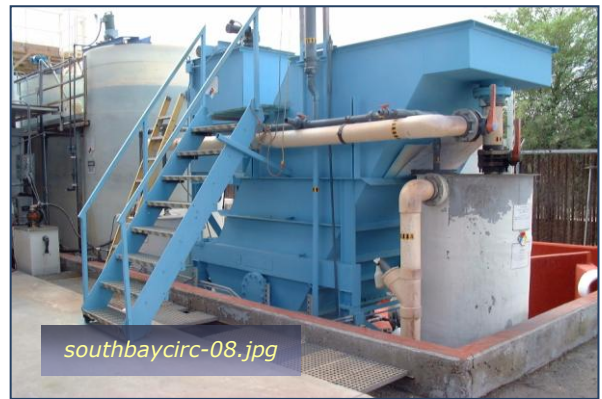
Photo #6: IWTP Lamella Clarifier Taken By: Greg V. Arthur Date: 08/11/09
