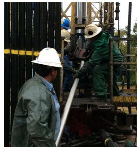
Figure 14: Installation of nano-laminated clad pup joint to improve corrosion performance and reduce rod wear.
