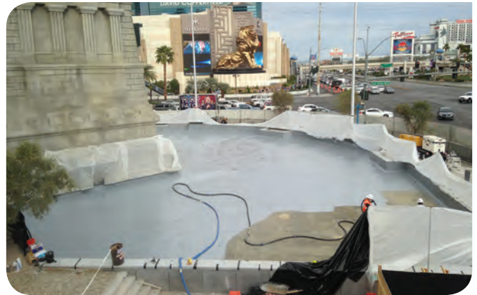
Wielding a Probler P2 spray gun for the first time, the crew from Water FX started the polyurea system with a mist coat of primer. That was VF 20, which was then backrolled.
