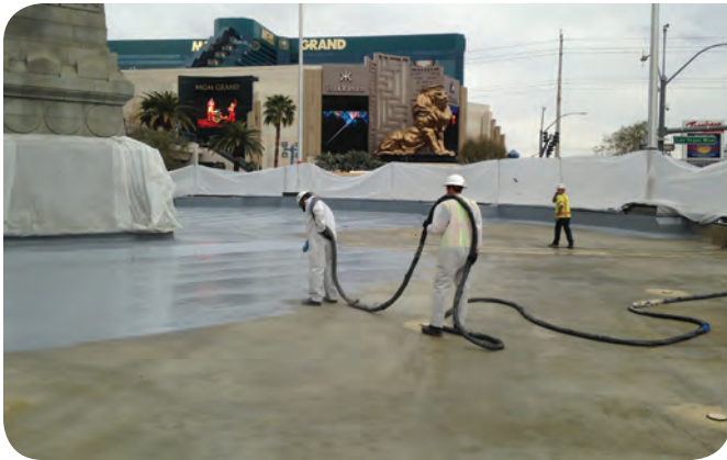
When the lagoon at the New York-New York Hotel & Casino in Las Vegas started leaking, the owners decided to demo it and start over. That included a 9,600-square-foot (891.9 m 2 ) caulk and coating job.
