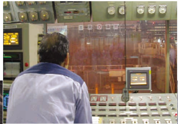
Sizing Mill Operator Room
