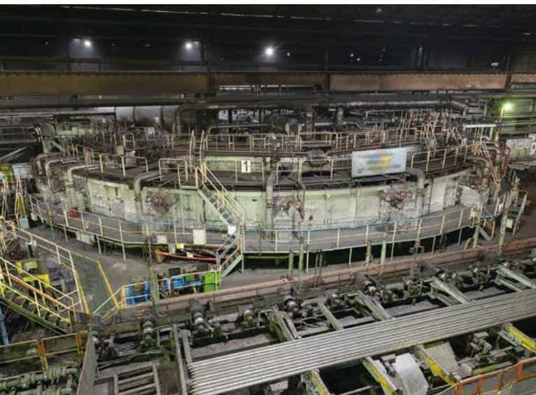
Regenerative burner type rotary hearth heating furnace
