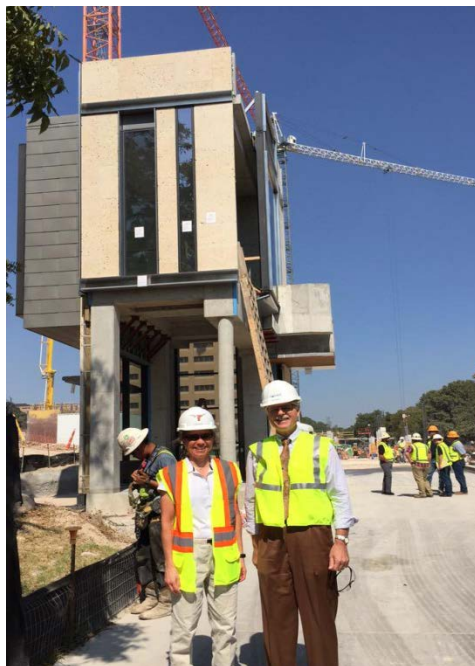
Above: Wood (left) at the Engineering Education and Research Center (EERC) construction site with project partners.
