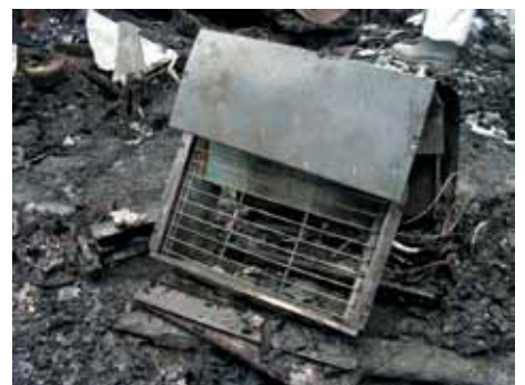
THE HEATER AND CYLINDER FOLLOWING THE FIRE.
