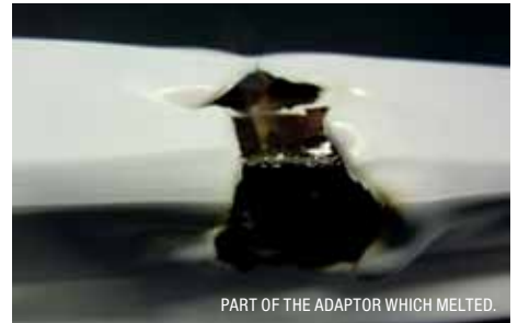
PART OF THE ADAPTOR WHICH MELTED.
