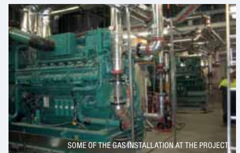
SOME OF THE GAS INSTALLATION AT THE PROJECT
