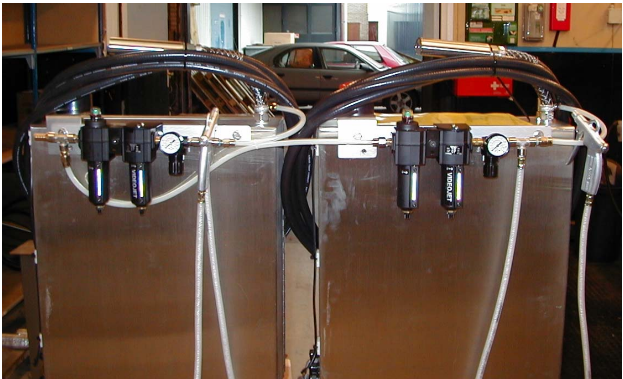
Figure 19. Two printers where air-reducers are connected.
