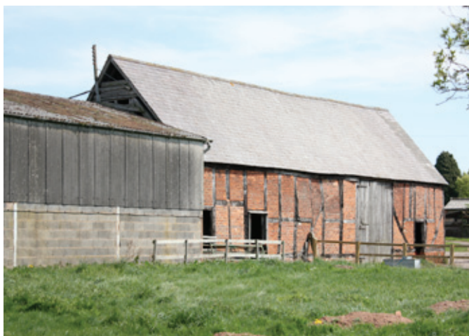
A timber-framed two-storey cow house of 17th or early 18th century date. Photo © Bob Edwards
