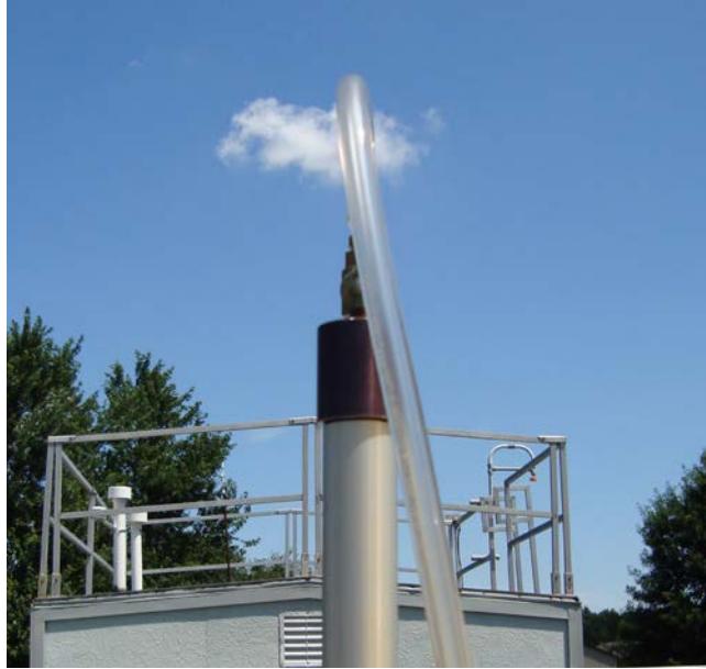
Figure 20. Flow Audit Adapter Installed.
