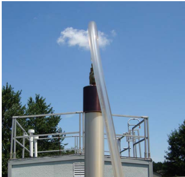
Figure 19. Flow Audit Adapter Installed.
