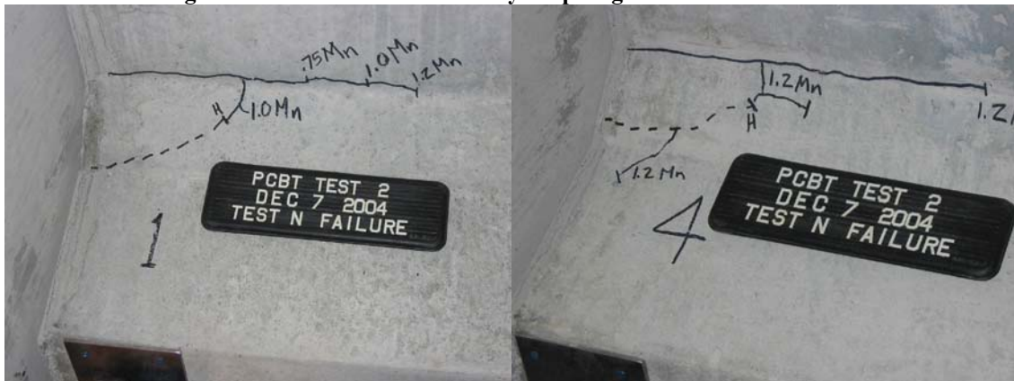
Figure 31. Cracking in End of Girders for Test 2
