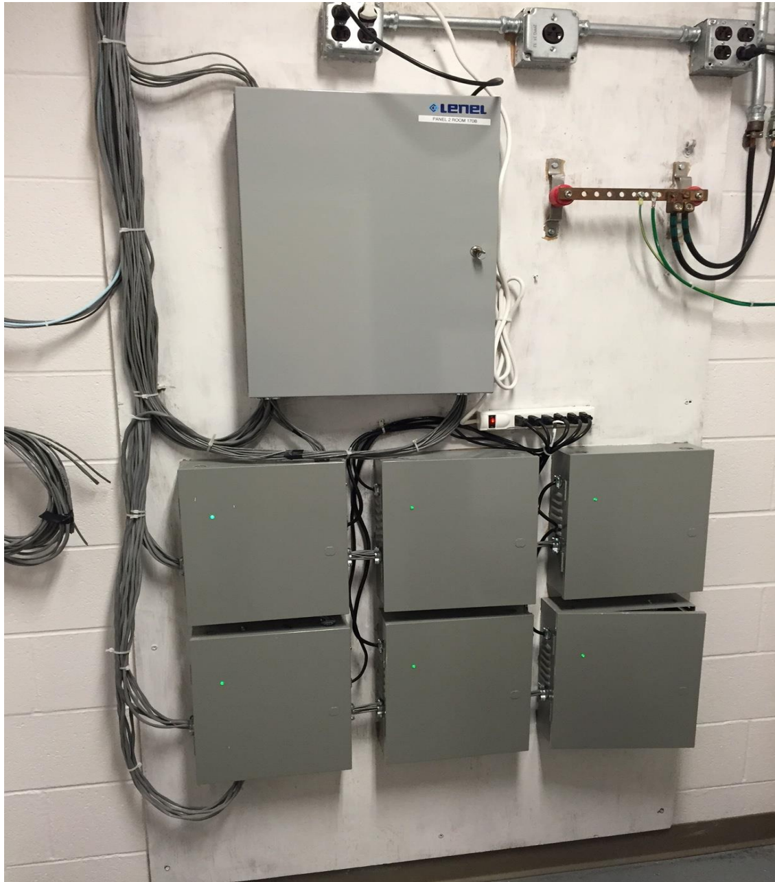
Panel with Power Supply
