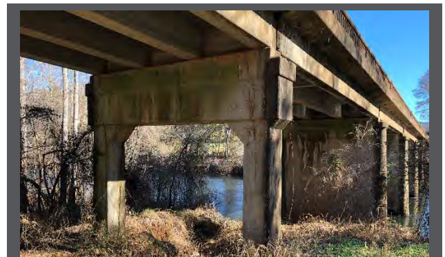
Bridge TIR for SR 40 over the Ocoee River in Polk County, TN
