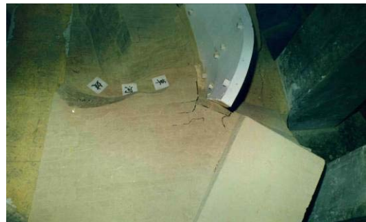
Photo 6. The failure mode of left abutment
