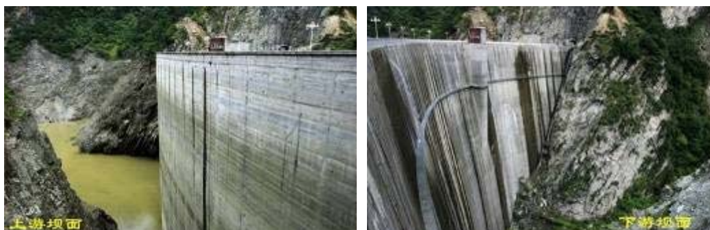
Photo 1. Little earthquake damage of the Shapai RCC arch dam after after Wenchuan earthquake
