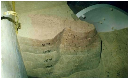
Photo 5. The failure mode of right abutment
