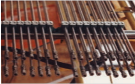
Instrumentation pipework made of stainless steel
