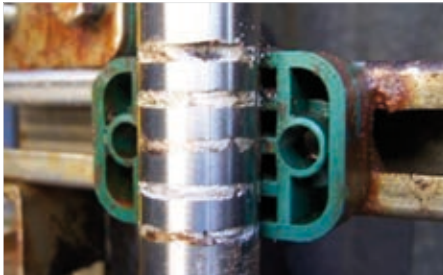
Crevice corrosion formed under a regular plastic clamp
