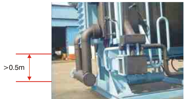
NPSH (R) maintained
