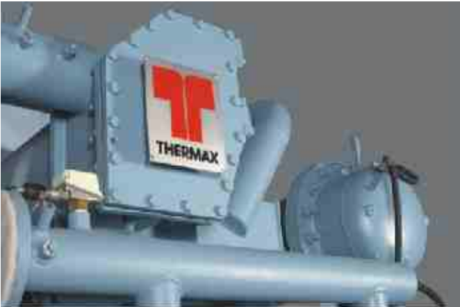
The HTG, LTG, Condenser
