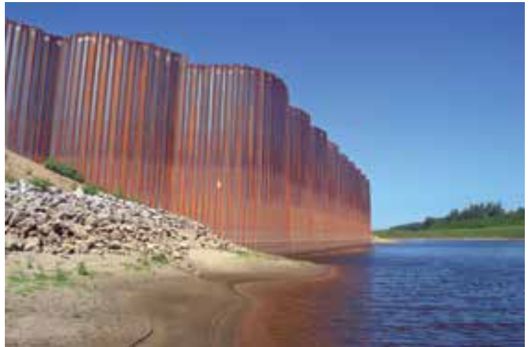
Cates Landing Intermodal Ports Authority, Tiptonville, TN (Shown during construction prior to installation of face beam and fenders.)
