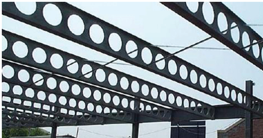
Fig. 2-13. Typical erection bracing for cellular beams (similar bracing used for castellated beams).
