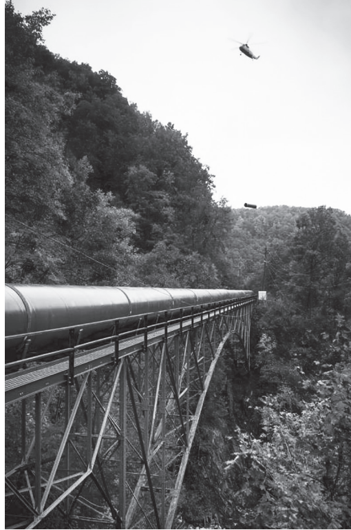
Figure 1-1 Steel pipe penstock on bridge
