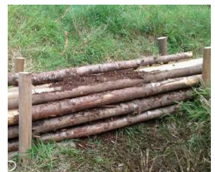
A constructed down log in a crib in Coos Bay, OR. Photo: Yankee Creek Forestry
