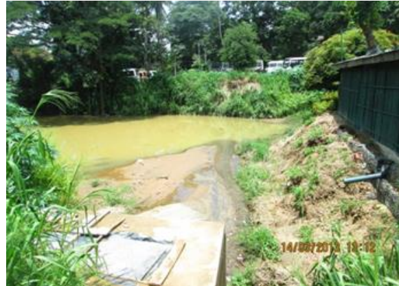
Figure 3. Red Culvert Lower
