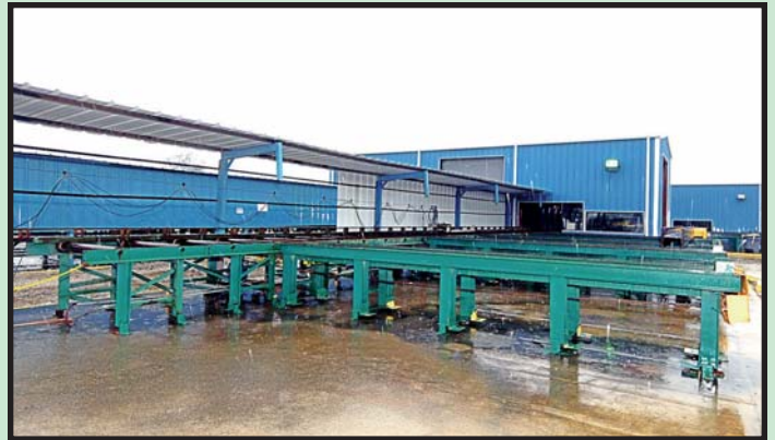
PUNCH LINE OUTPUT CONVEYORS
