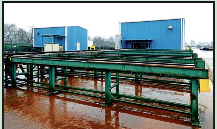
CONTROLLED AUTOMATION PUNCH LINE INPUT CONVEYOR
