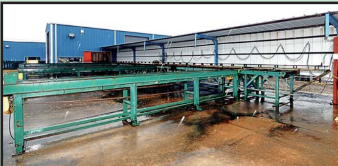
DRILL LINE OUTPUT CONVEYORS
