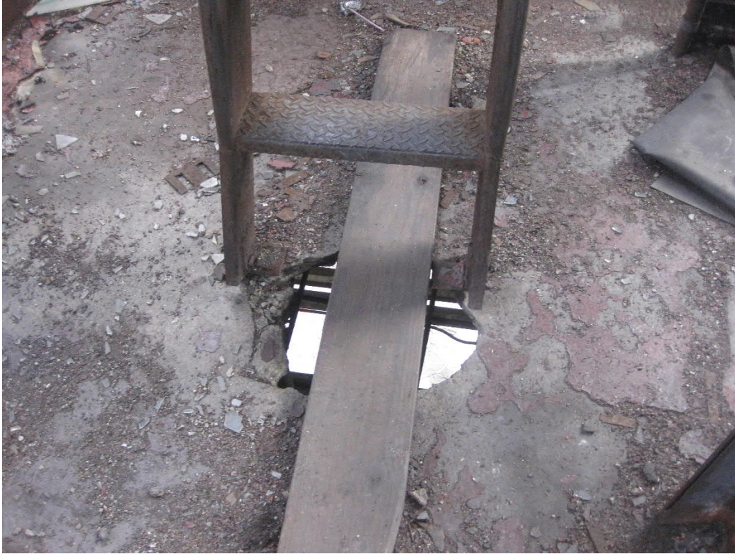
Photo #18 – Hole in 7 th floor slab
