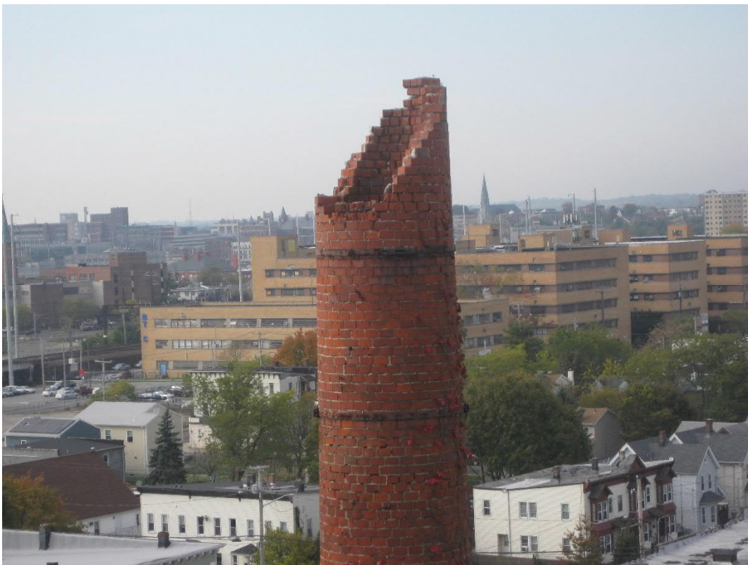
Photo #25 – Damage, loose bricks and steel bands at top of stack
