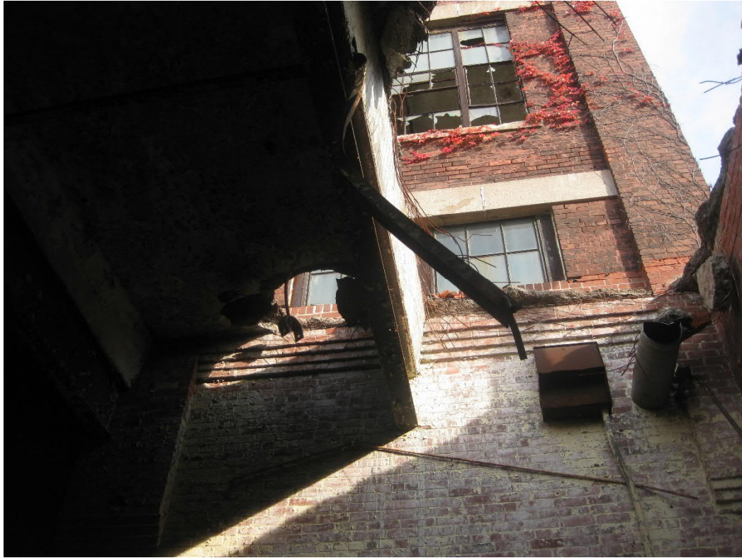
Photo #2 – Failure at low roof deck at second floor level
