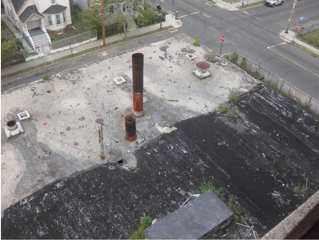
Photo #16 – Failed roofing at low roof
