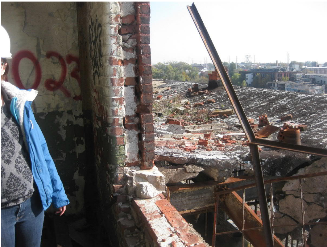
Photo #13 – Damaged window frame, sill and jamb
