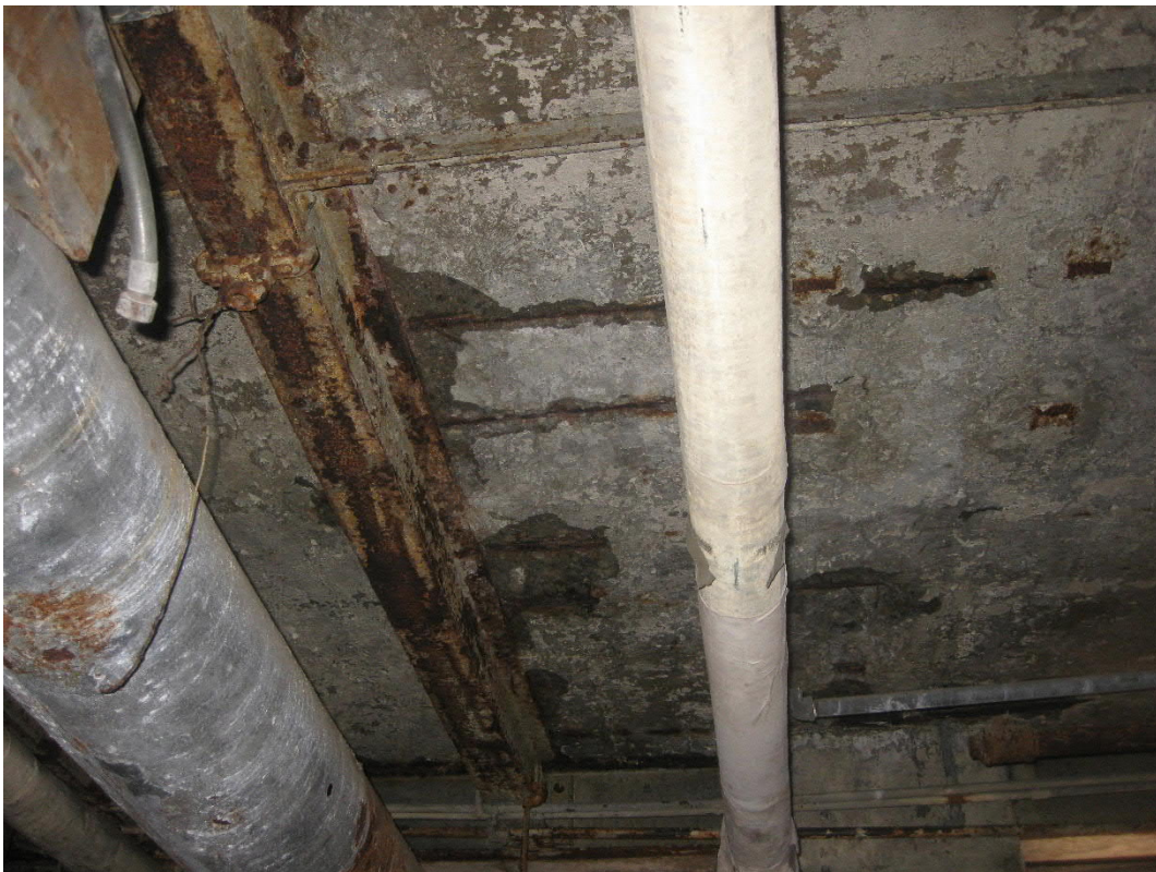
Photo #9 – Concrete deck damage and rusted steel at second floor
