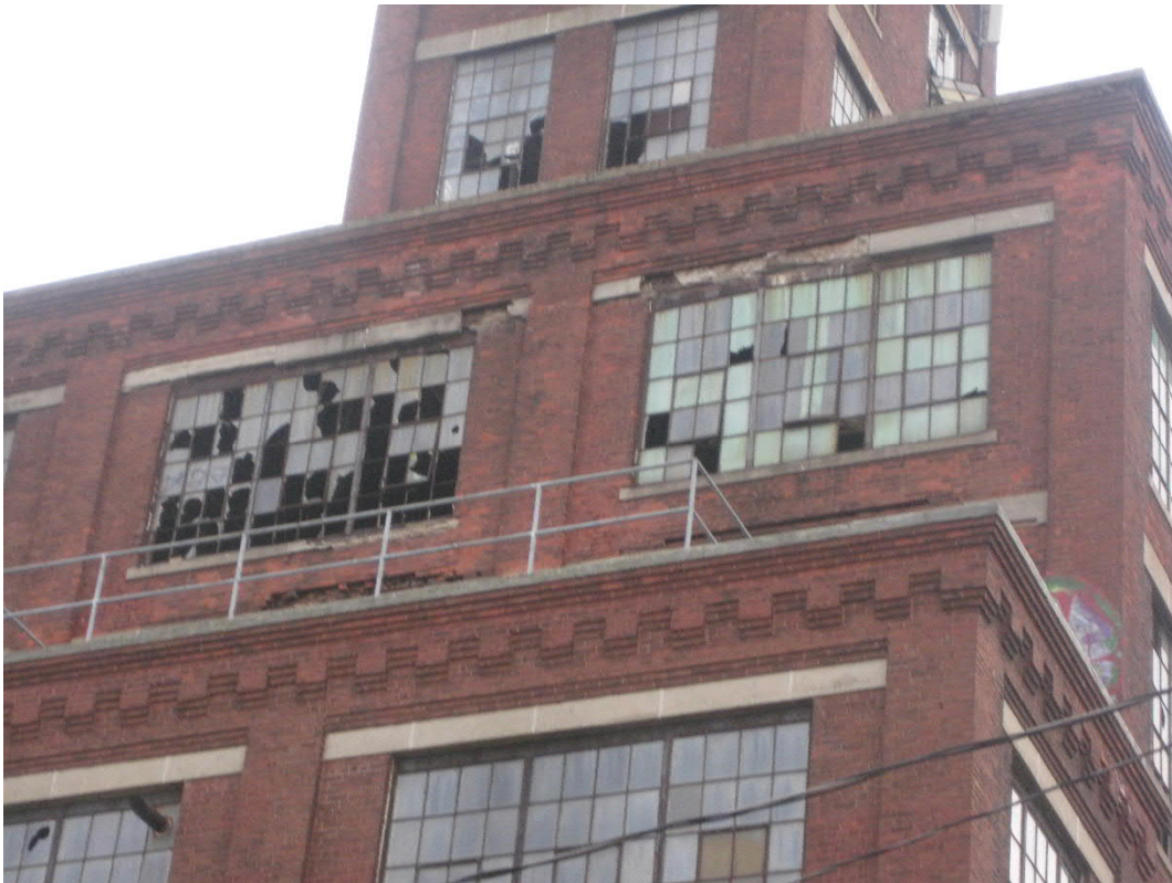
Photo #21 – Damaged concrete lintels at north face
