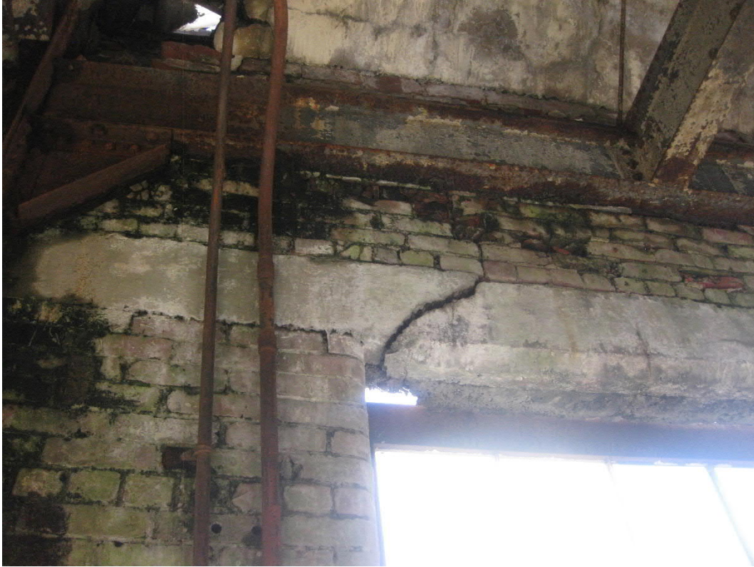
Photo #14 – Failed concrete lintel
