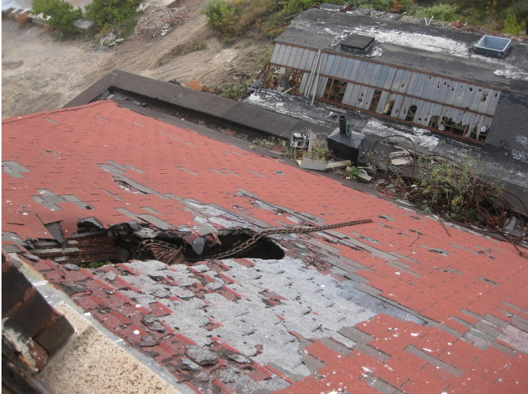
Photo #6 – Hole in sloping roof deck on south side
