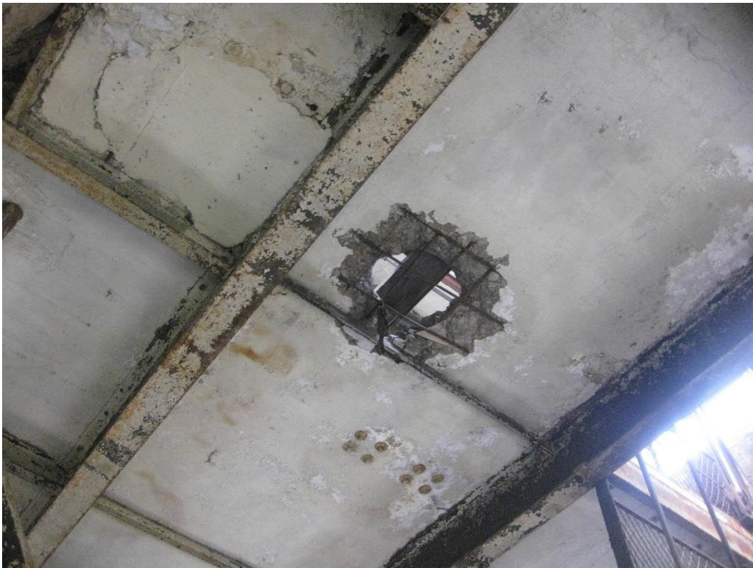
Photo #19 – Hole in 7 th floor slab
