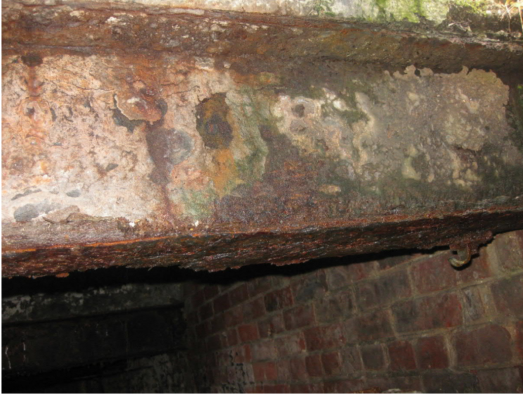
Photo #10 – Rusted framing at first floor
