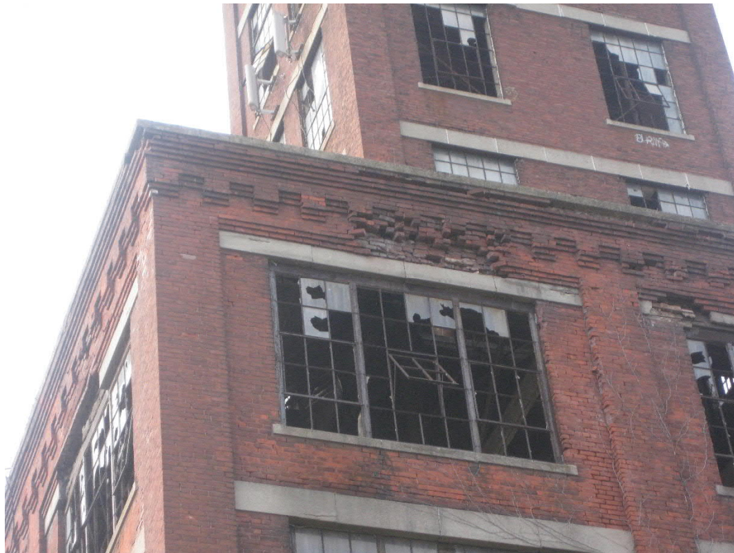
Photo #22 – Damaged brick at east face
