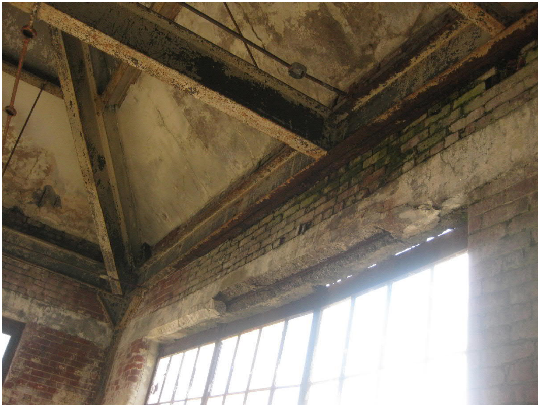
Photo #15 – Damaged concrete lintel
