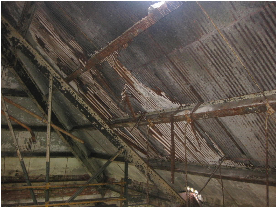
Photo #7 – Failed metal deck and rusted framing on north side of sloping roof
