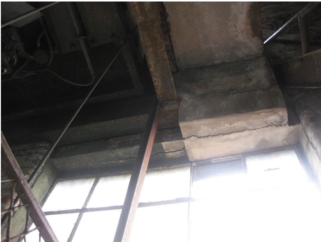
Photo #11 – Cracked lintel at window head
