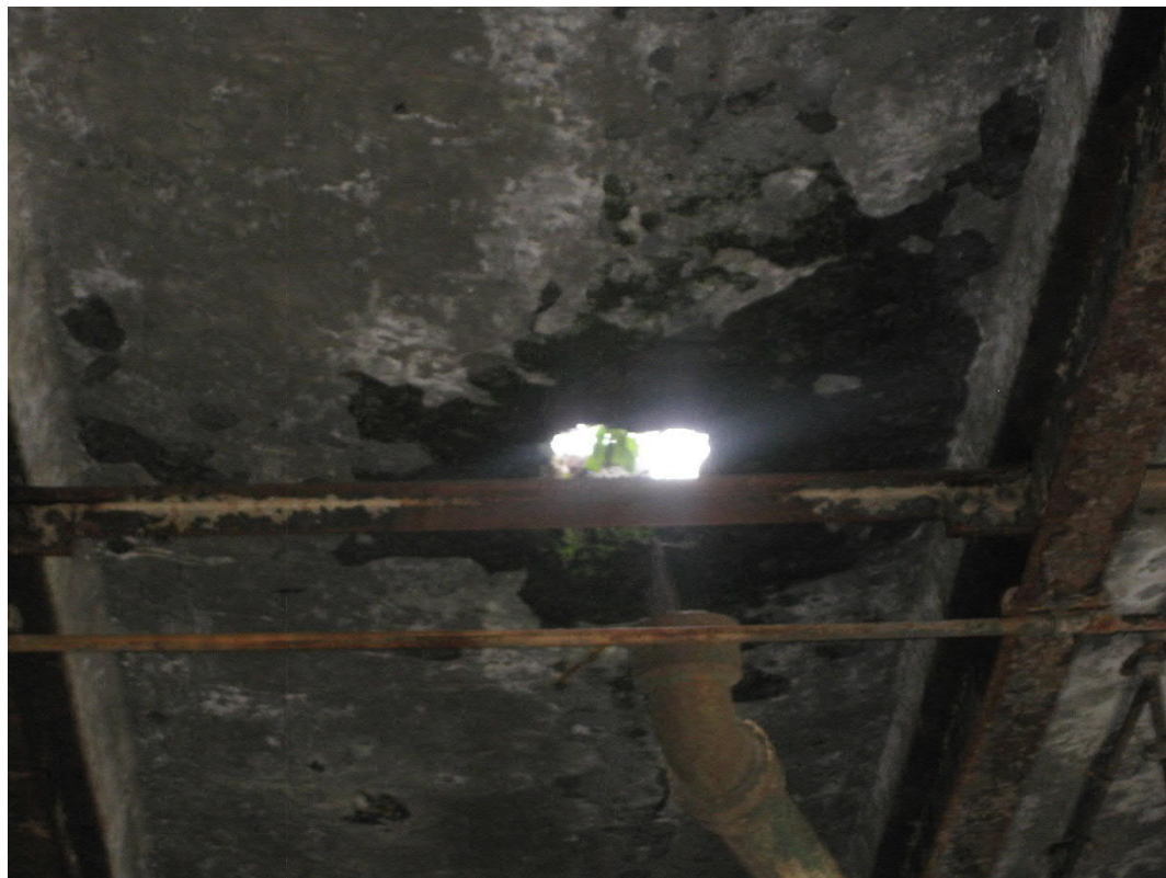
Photo #23 – Roof deck damage at removed drain pans
