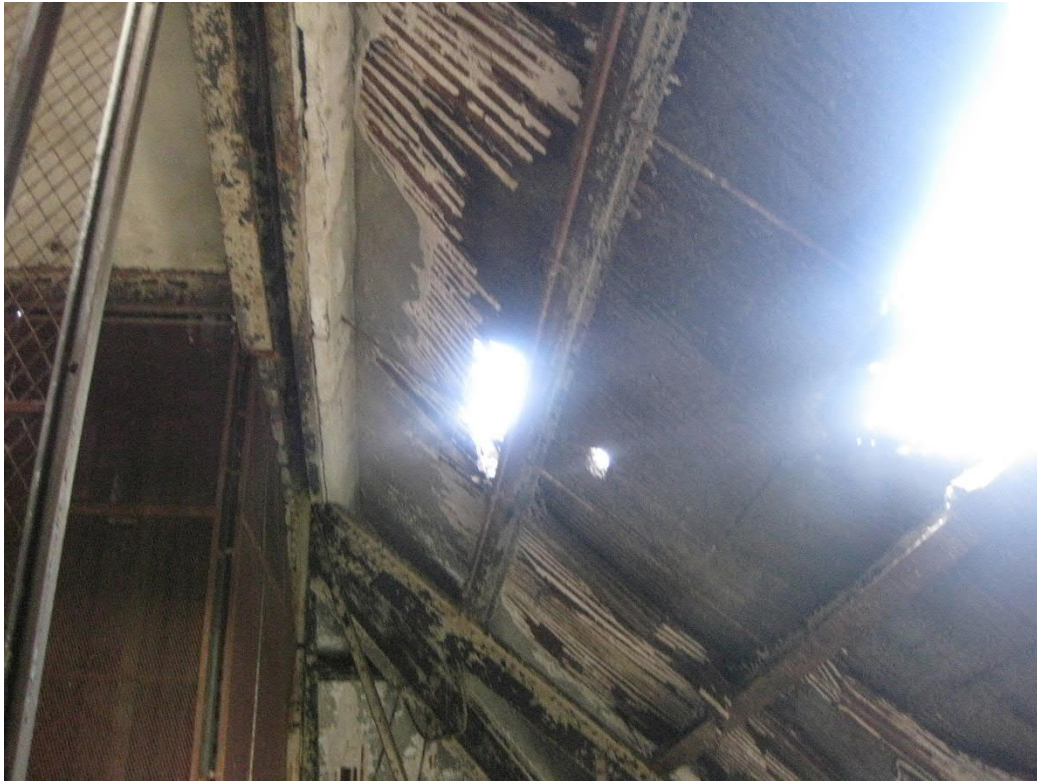
Photo #4 – Failed sections of sloped roof at north side
