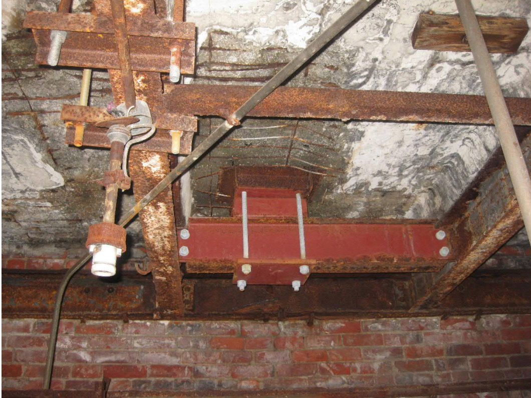
Photo #8 – Spalling concrete roof deck and rusted framing at upper roof
