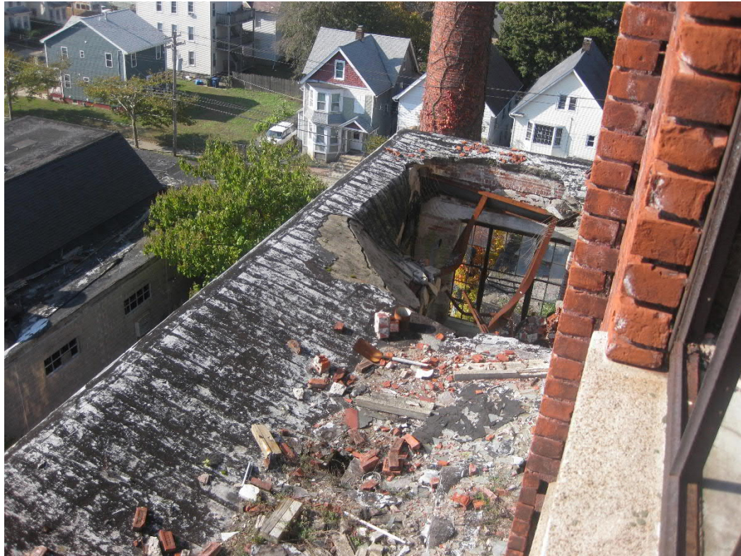
Photo #3 – Failure at low roof at fifth floor level
