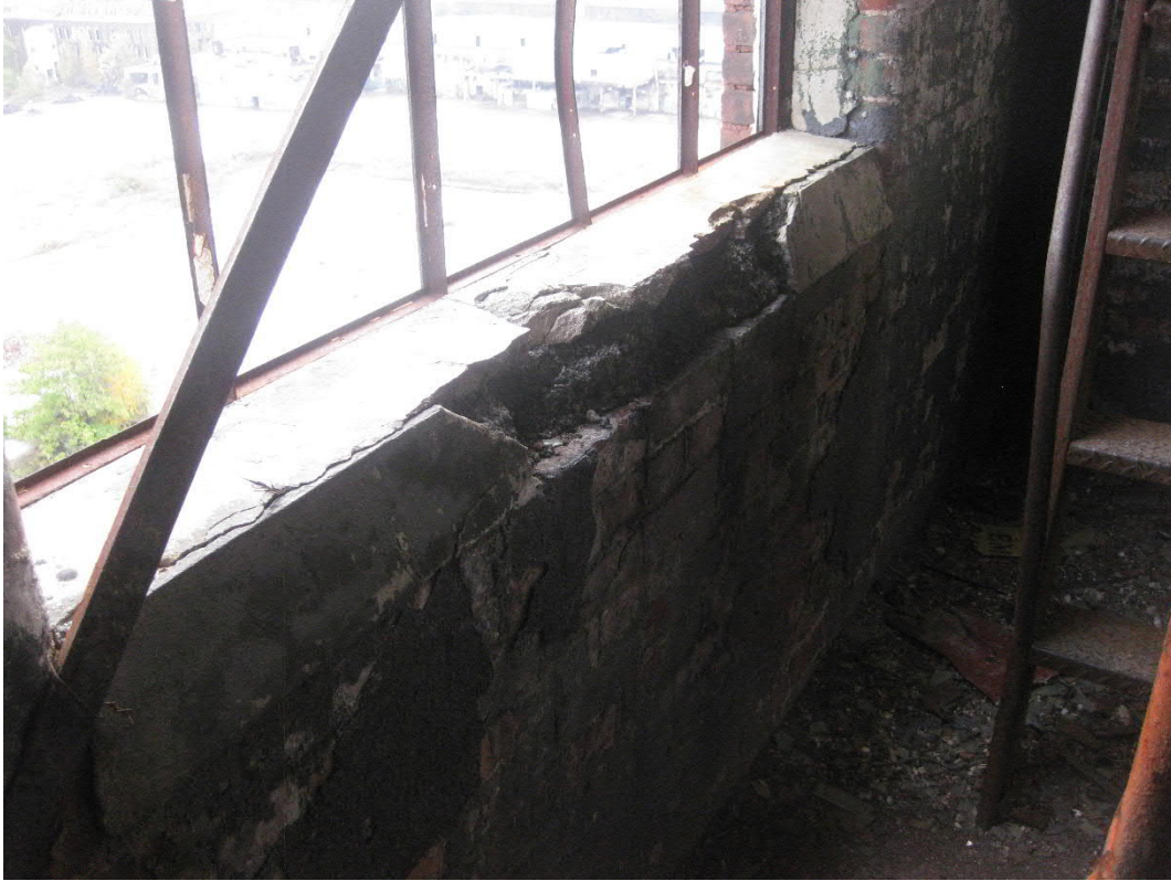
Photo #12 – Damaged window sill and frame
