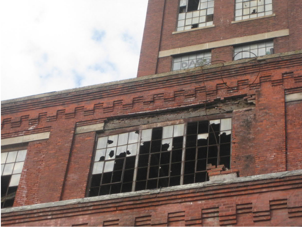
Photo #20 – Damaged concrete lintel at south face
