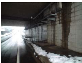
Figure 3. Water leakage from the joint.
