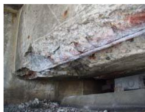
Figure 4. Degradation of the girder ends.
