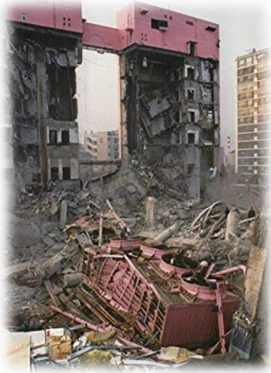
Sampoong department store collapse due to overload (Seoul, South Korea, 1995) 502 killed people 937 injured
