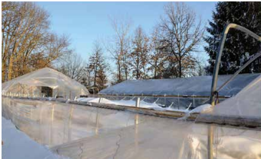
Fig. 2. Collapsed greenhouse caused by an uneven snow load
