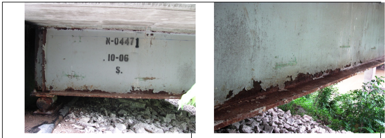
Figure 4.2 Example of System S Coating with Early Failure, End-span of Fascia Girder.
