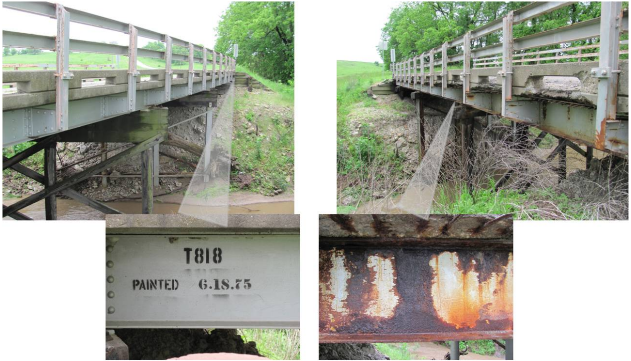
Figure 4.7 Example of the Effects of Deck Drainage on Coating Condition.
