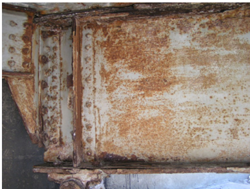
Figure 3.5 Example Photograph for Interior Sections of a Bridge with Coatings in Very Poor Condition.
