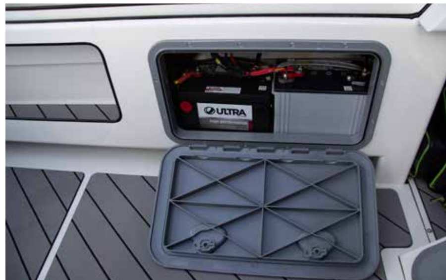
Above: The batteries are kept in the port side gunwale, protected from the elements; The well laid out helm station is dominated by a 12' Garmin sounder/plotter.
