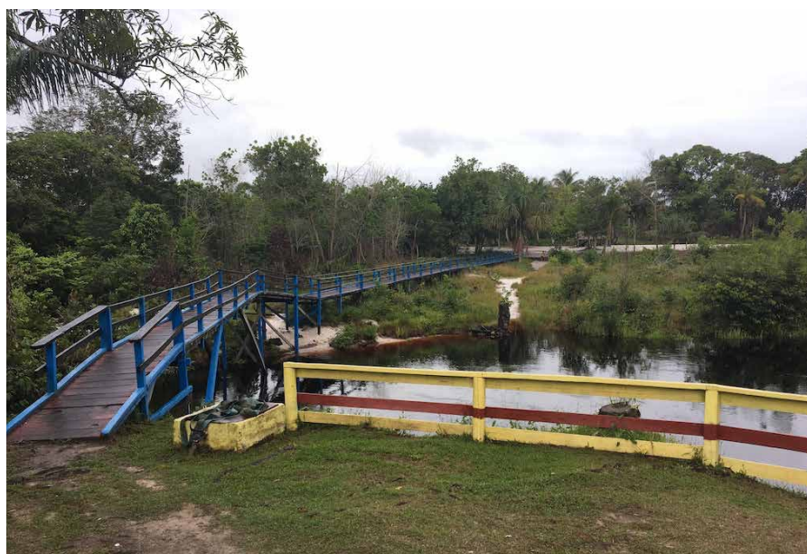
Figure 61: Bridge that was covered after a flood in Moraikobai
