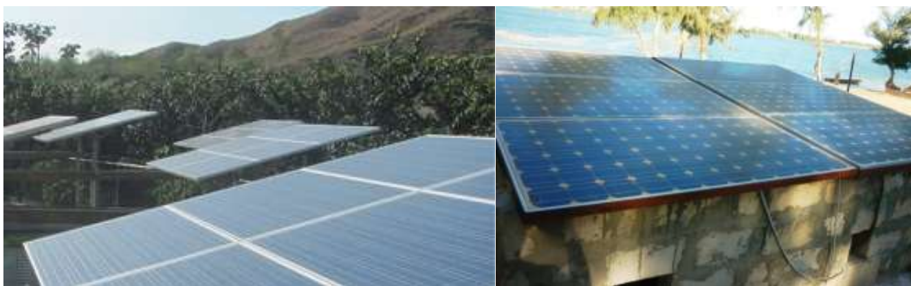
Figure 32 A and B. A. Photovoltaic panels above the fish tanks at Lashto Fish Hatchery Haiti (2012). B Solar panels on roof of catfish and tilapia hatchery Senegal (2013)
