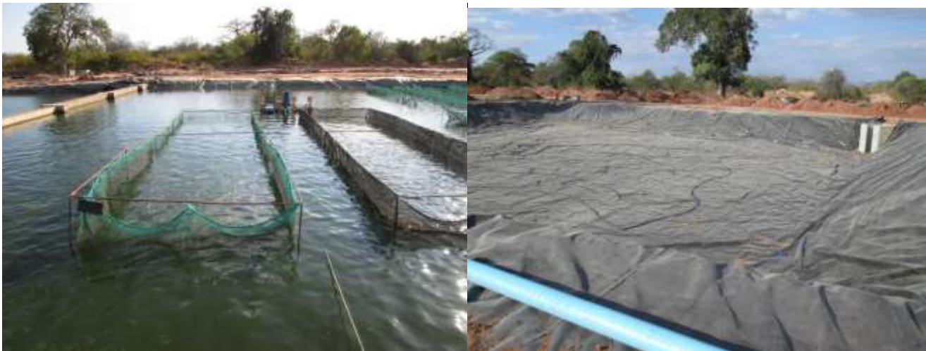
Figure 18a and 18b a. Broodstock ponds with hapas and paddlewheel aerators b. Installation of piped compressed air aeration system.
