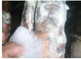
Figure 6. Leaking detected during pressurized test
