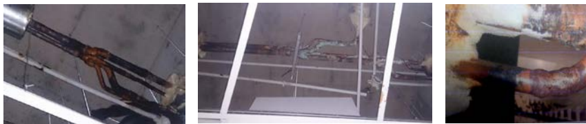
Figure 7. Improper installed pipe due to poor workmanship
