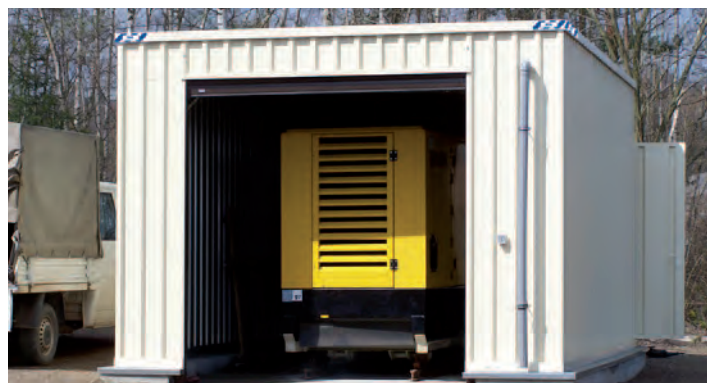
Power generator housing at a mine
