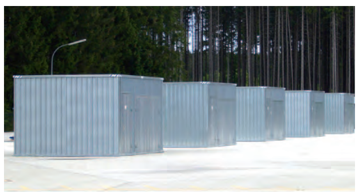
Gas distribution units
