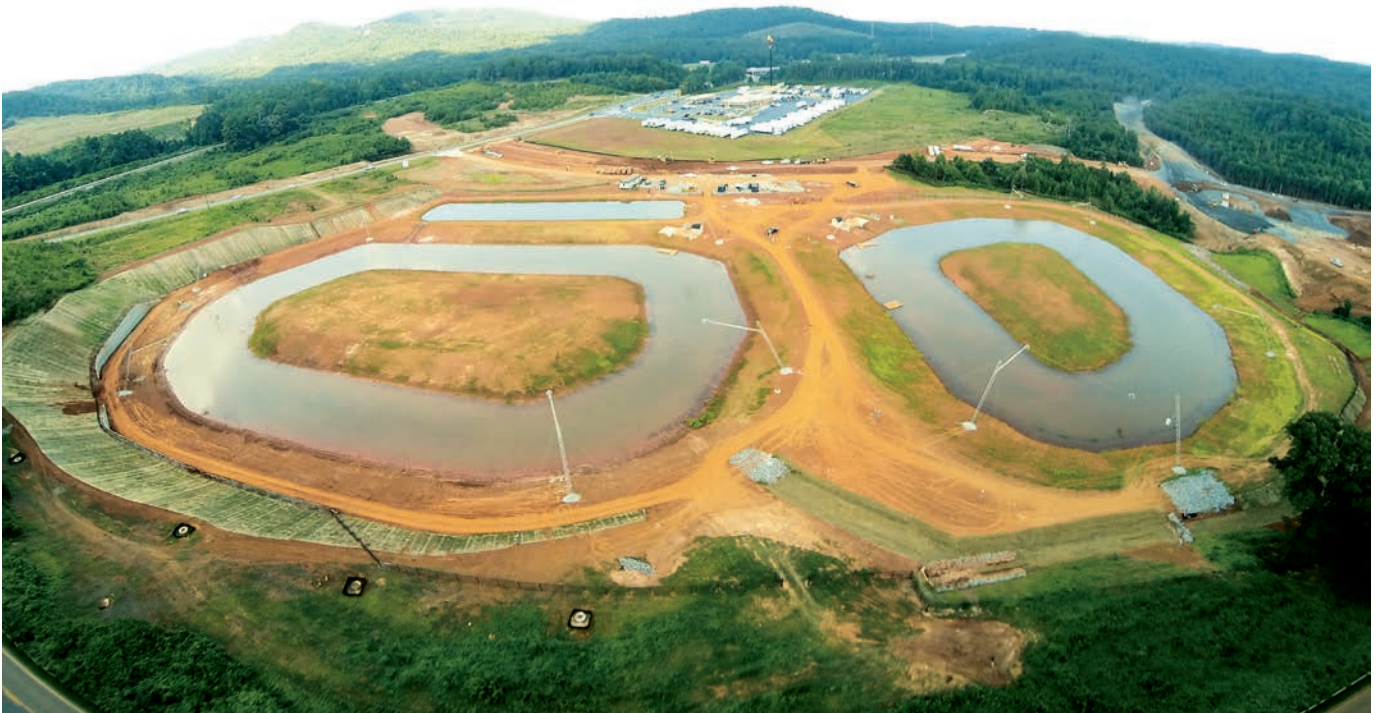
PHOTO 2 Terminus Wake Park prior to subgrade prep and dewatering, looking east. Lake 2 is on the right, Lake 3 is on the left, and Lake 1 is just beyond Lake 3.
