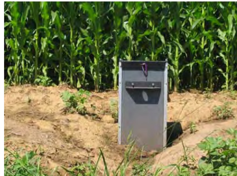
Water control structure placed at the end of a drainage system.
