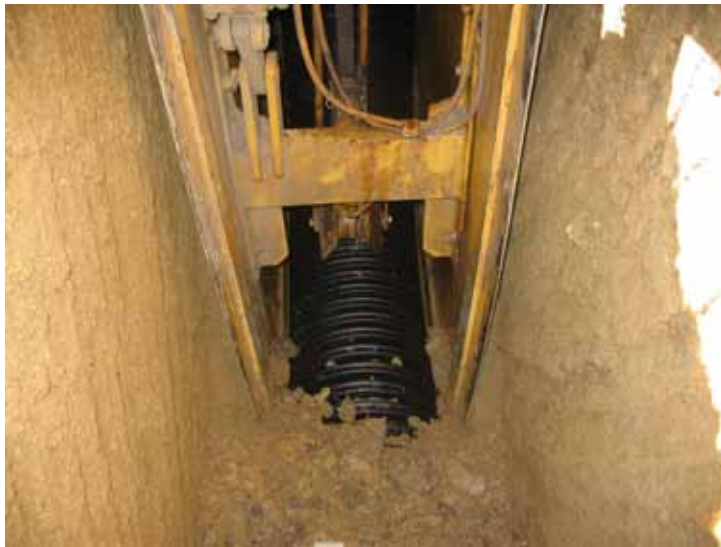
Close up of corrugated plastic tubing being installed by a trencher type tile machine.
