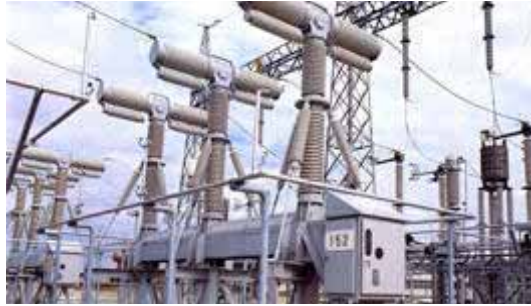
Gambar X.8 VCB (Vacuum Circuit Breaker) Out Door 145kV
