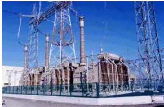
(c) Transformator 1000MVA
