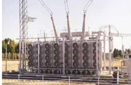
(b) transformator 4500MVA
