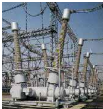
Gambar X. 4 (a) Gas Switchgear Combined (GSC) 550kV
