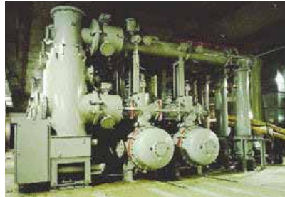
(b) Gas Insulated Switchgear (GIS) 300kV
