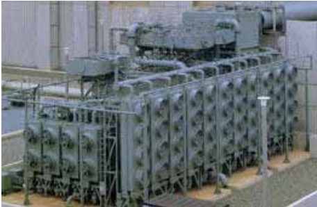
(a) transformator 1100MVA
