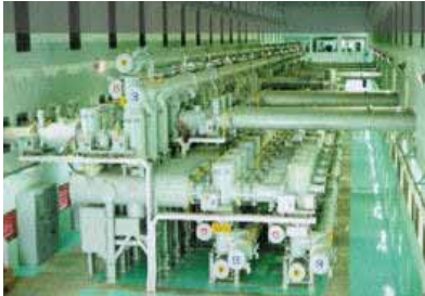
(a) Gas Insulated Switchgear (GIS) 550kV
