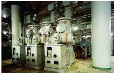
(c) Gas Insulated Switchgear (GIS) 84kV
