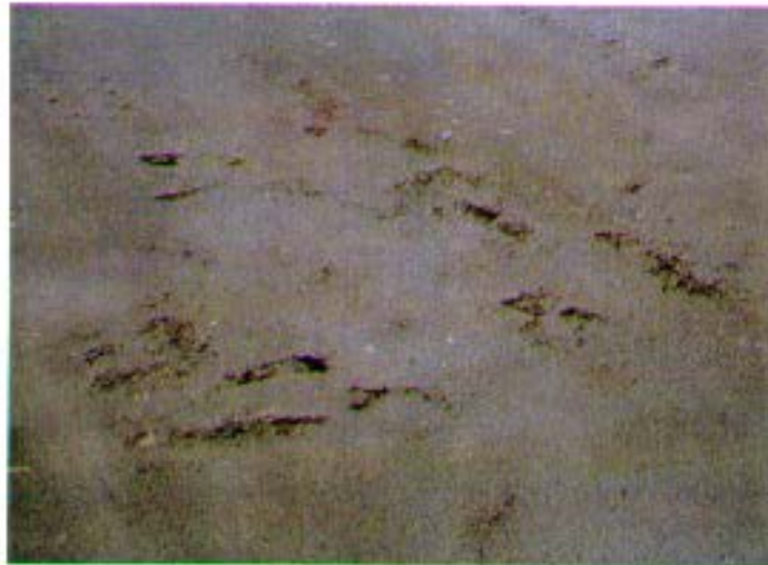
Figure 8 - SAF layer tearing from screeder
