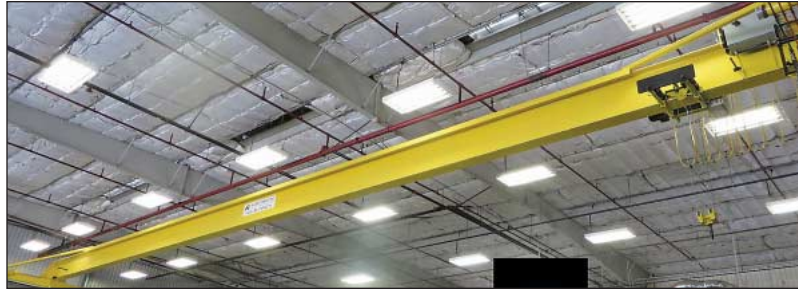
2 Ton x Approx. 77' Span x Approx. 100' Long Free-Standing Overhead Bridge Crane
