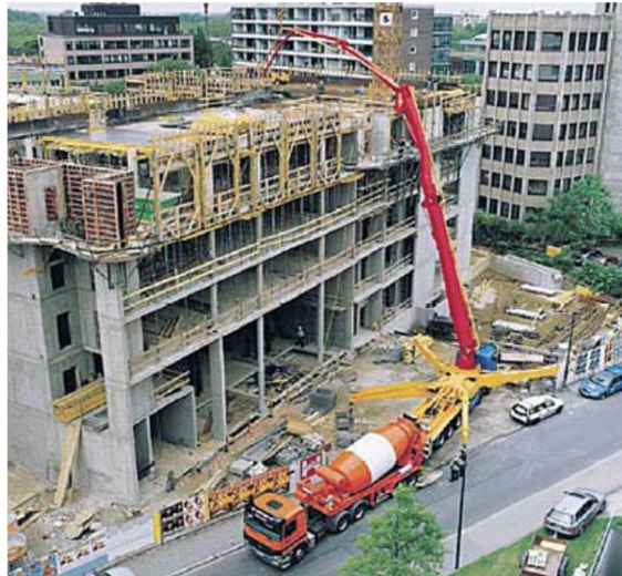
Figure 11. Programmable, articulated-boom machine for the pumped delivery of fresh concrete [source: Saidi et al. 2008].
