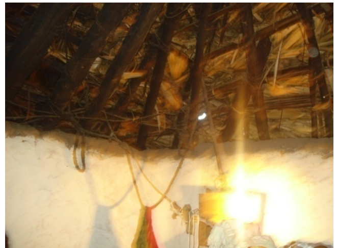
Fig. 14 Lack of air outlet at ceiling level in existing hut
