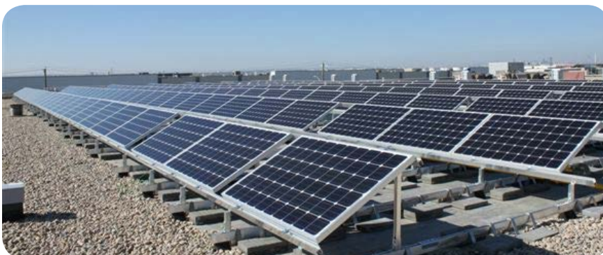
A solar system sits atop the roof of our Calgary location.
