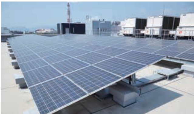
Solar Power Generation Facilities at Hikari plant
