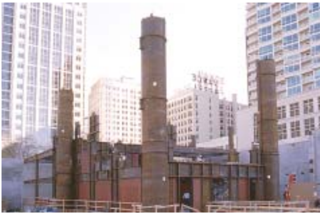
Key to the steel-plate, shear wall core are large-diameter pipe columns filled with 10,000-psi concrete.
