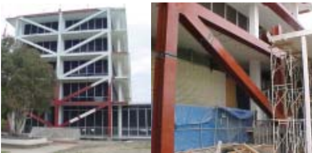
Builders Steel Project-Costa Mesa City Hall, new framework and closeup of connections.
