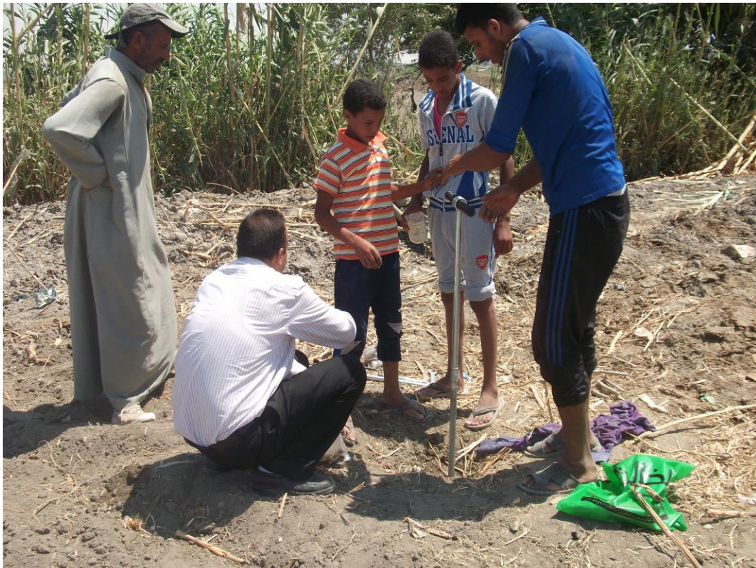
Photo 3: Drilling test boreholes to investigate subsurface section at the proposed site for construction of wastewater treatment plant (profile No. 1)
