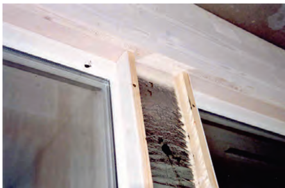
Picture 3: Window frames are covered with custom sized VIP. The VIP is protected by a wooden box.
