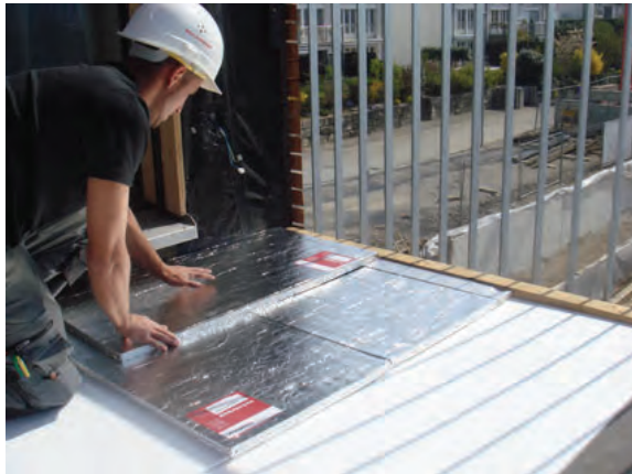
Picture 2: Roof terrace with double layer VIP. The complete insulation amounts to 24cm rock wool, 4cm VIP and 3 – 6cm foam glass.
