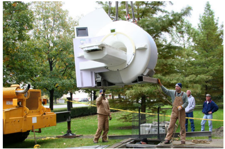
The 3T Allegra Headscanner is moved by crane to the Beckman basement opening on the north side of the building.
