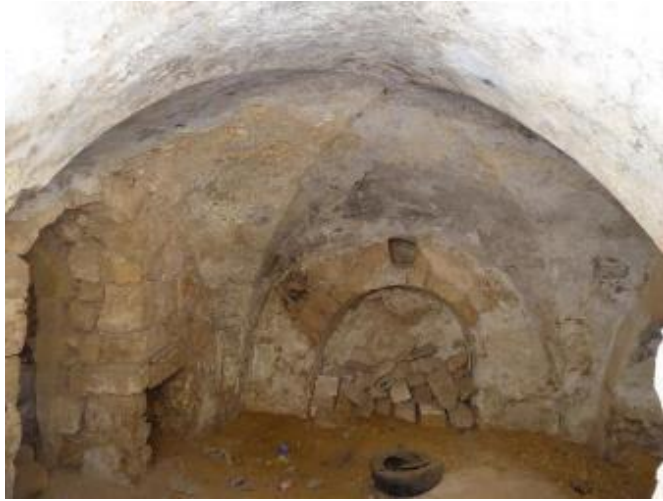
Image 10 Hebron's old town: cross vault in an abandoned building. We can see the importance of corners in load bearing issue.
